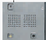
Controls embedded into the wall.
